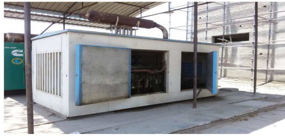
Figure 4: Diesel Generator (125KVA, Crompton Greaves)
